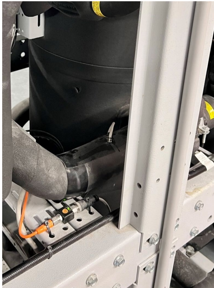
Figure 19 High pressure expansion valve CO 2 temperature sensor and IFM converter module.
