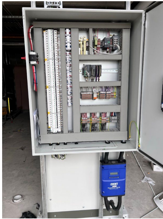
Figure 20 Electrical board- Electrical breakers, PLC and DENT power meter.
