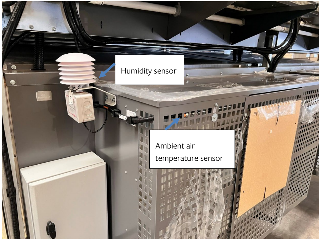
Figure 14 Ambient air temperature and relative humidity sensor.
