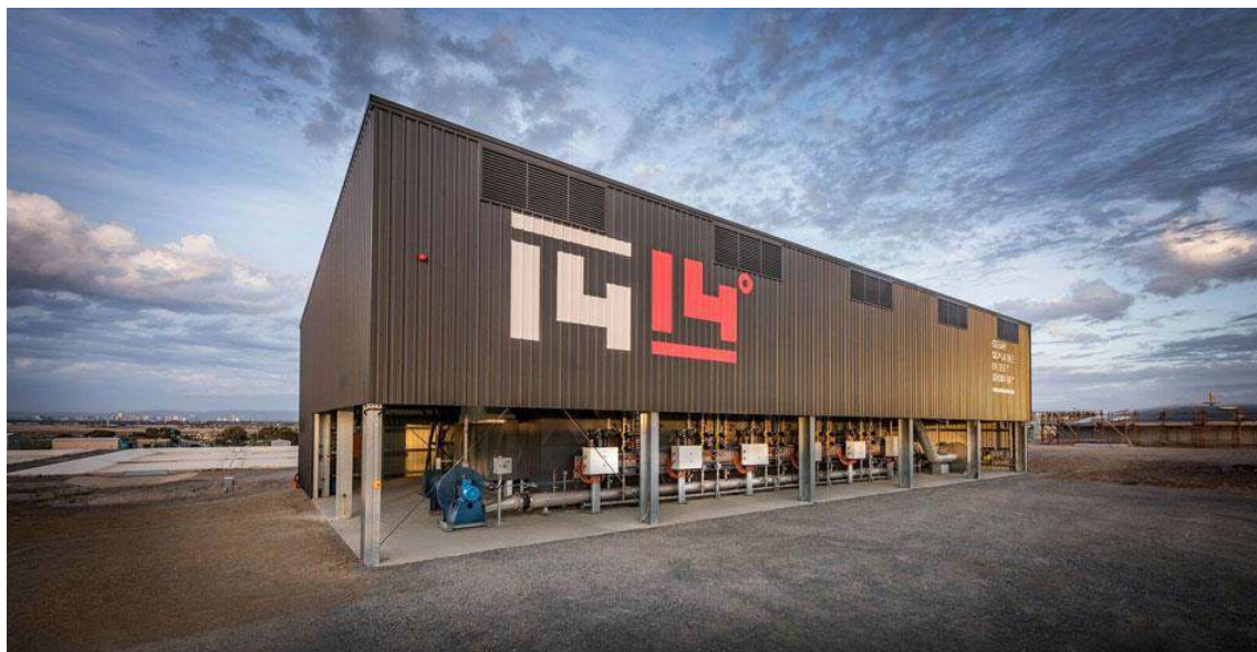
Figure 53. 1414 Degrees' biogas thermal energy storage system [201].
