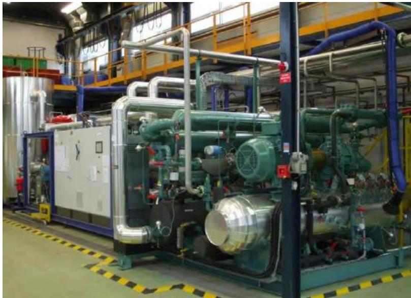
Figure 49. Picture of the Johnson Controls /EDF heat pump [150].
