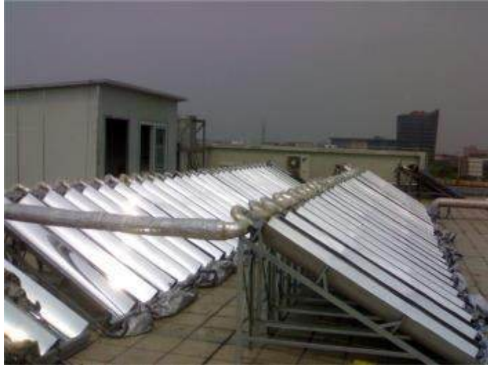
Figure 51 Photograph of the evacuated tube air heater [181]
