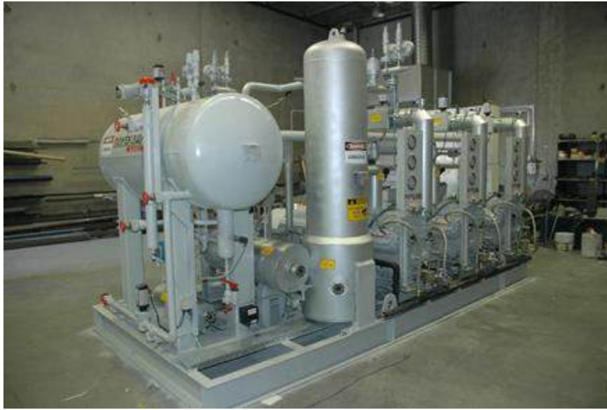
Figure 43. Example of an ammonia high-temperature heat pump manufactured by Mayekawa [144].
